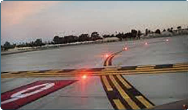
Figure 14-35. Runway Entrance Lights (REL).
